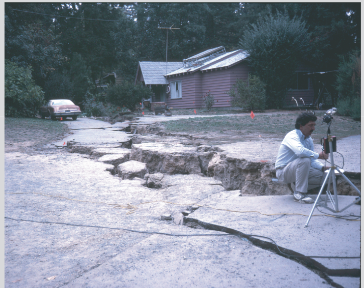
Figure 4B. View NW at structure damaged by shaking-induced fissuring during Loma Prieta earthquake. Location of photo shown on Fig. 4A.
