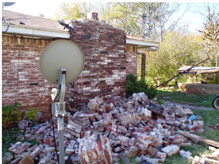
Damage caused by the magnitude 5.7 earthquake near Prague, Oklahoma, November 6, 2011. Unreinforced stone and brick buildings (especially chimneys) are some of the most vulnerable structures in any earthquake. Image credit: Brian Sherrod, USGS 10
