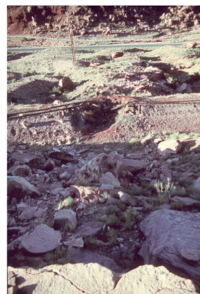
Figure 2: Additional Rock-fall damage to railroad tracks on the west side of the Colorado River just west of the Portal
