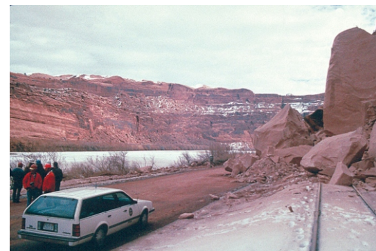
Figure 1: Rock-fall damage to railroad tracks on the west side of the Colorado River just west of the Portal.
