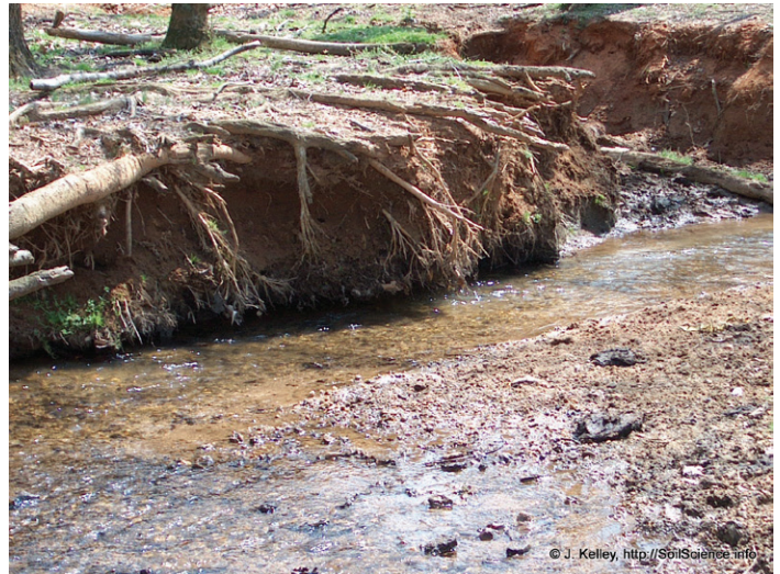
Streambank erosion can be a major contributor of sediment to downstream waters.
