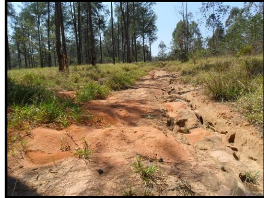
Figure 2: Erosion on forest roadway
