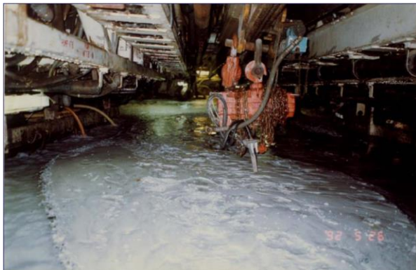
Figure 1: Flow of Silt Laden Water under pressure due to puncturing of Shear Zone by TBM at HRT-Dulhasti Hydro-electric Project, J&K, India
