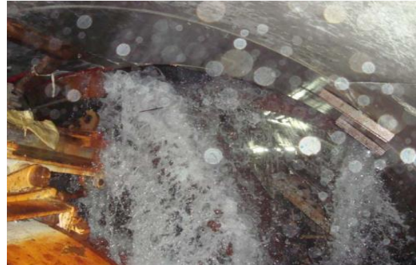
Figure 2: Water Ingress from segment number 1905 in HRT of Tapovan-Vishnugad Hydro-electric Project, Uttarakhand, India
