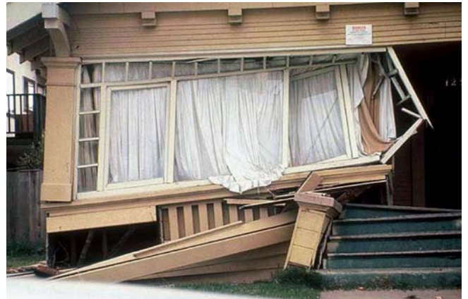
Wooden structure that shifted on its foundation during the 1989 Loma Prieta earthquake.
