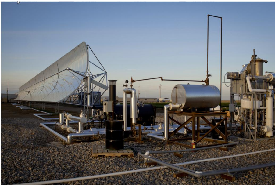
Solar Distillation Parabolic trough with heat transfer fluid (Solar FX—image from New York Times)
